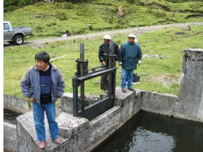
At the head sluice gate, where the water from the high Andes is collected for the main irrigation canal.
